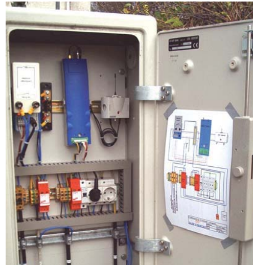
Remote Controlled Switching of Rectifier System with Main Power Supply Unit
