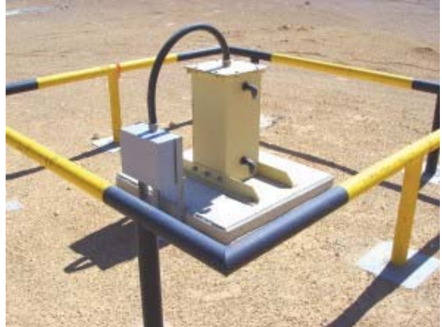
Anode Junction Box fixed with steel support mounted on concrete foundation at anode deep groundbed structure
